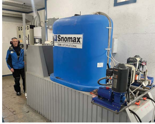
Mechanism where Snowmax enters HoliMont's high pressure water pipes for snowmaking.
