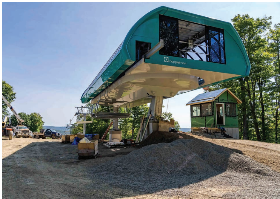
The old Mardi Gras lift has been shipped off to Corralco, Chile and the haul rope is spliced and up on the towers. The Mountain Crew has been building the new chairs and installing them on the cable. Electrical work is being done on the new lift houses. They are getting closer!
