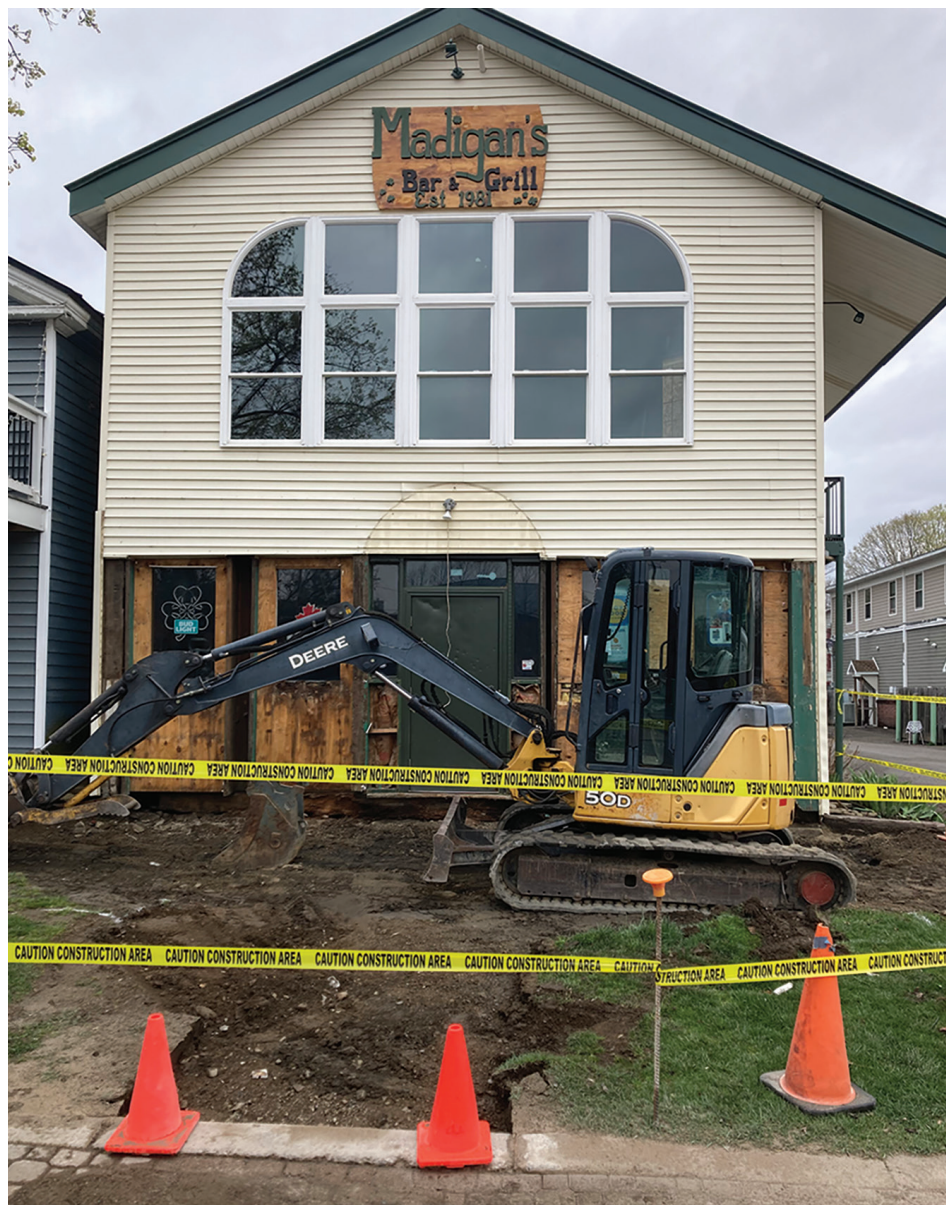
Patio deck construction underway at iconic Ellicottville hotspot. More to come in next couple weeks!
