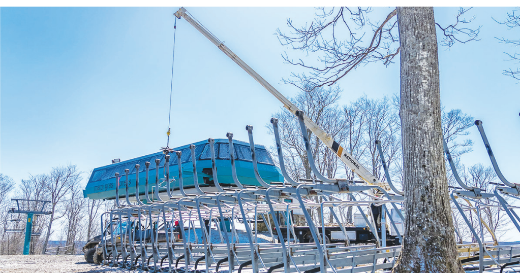
The Lift Team is hard at work removing chairs from Mardi Gras for part of its annual inspection. Even though winter is over, we're already preparing for next season! The Mountain Ops team continues to do clean-up work on the side of Mardi Gras. There's no shortage of work to do out there as we get ready for summer!
