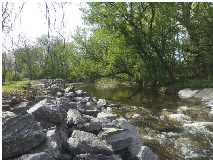
Ball creek stabilization project – heavy rock rip-rap and bank grading reduces water velocity, limits future erosion, reducing sediment and nutrients into the lake to limit fuel plant and algae growth.
